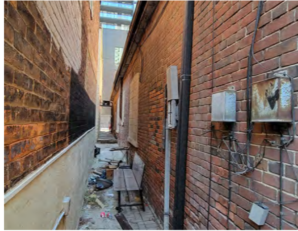
Figure 67: Areas of the east brick wall and concrete block infill is in defective condition (ERA, 2022).
