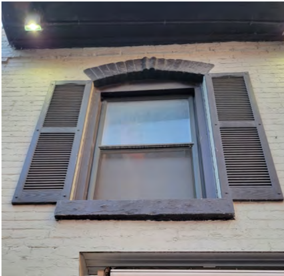
Figure 44: Wood shutters and sill in fair condition (ERA, 2022).
