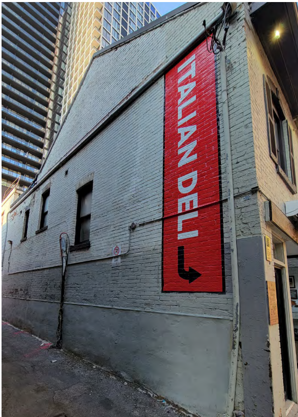
Figure 48: Parging at grade with exterior grade in poor condition (ERA, 2022).
