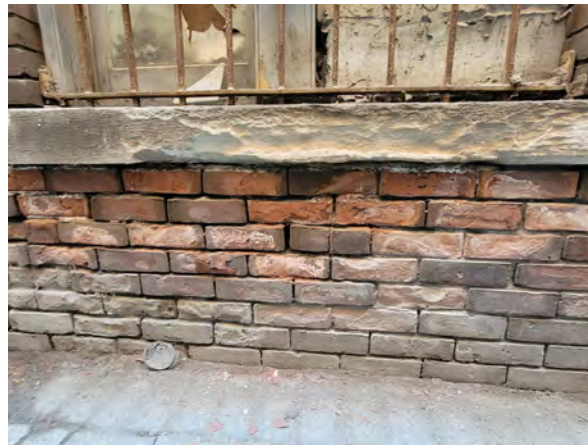
Figure 68: Spalled brick and damaged sills have no mortar, allowing water to enter the wall (ERA, 2022).
