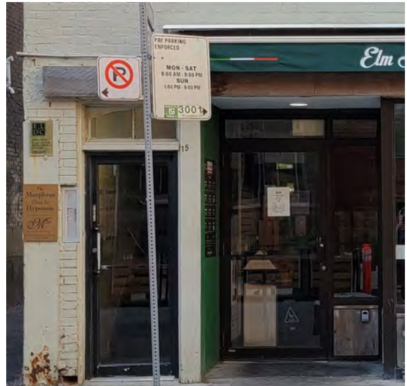
Figure 45: Second floor aluminium door with heavy steel angle and deteriorated brick in poor condition (ERA, 2022).
