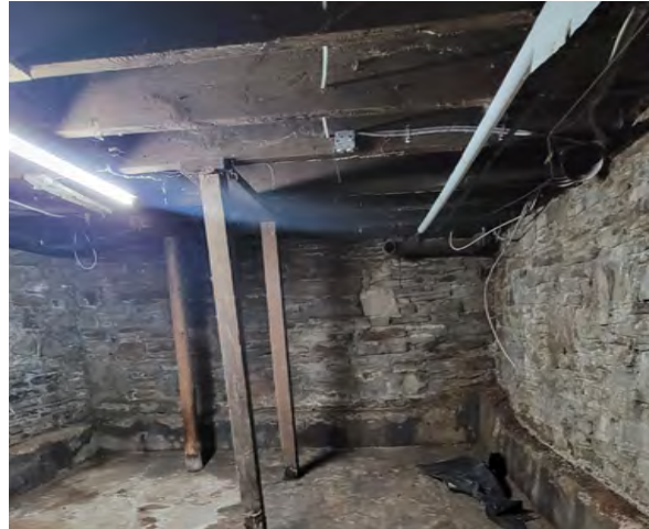
Figure 59: Wood posts shoring up sagging floor (ERA, 2022).
