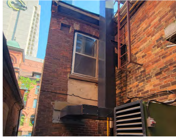
Figure 50: Open masonry with wood infill and windows ranging from poor to defective (ERA, 2022).
