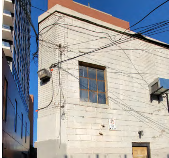
Figure 54: The south East corner is in poor condition (ERA, 2022).
