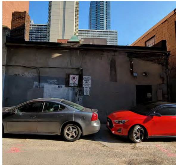
Figure 73: Chimney and corner brickwork are in poor condition (ERA, 2022).
