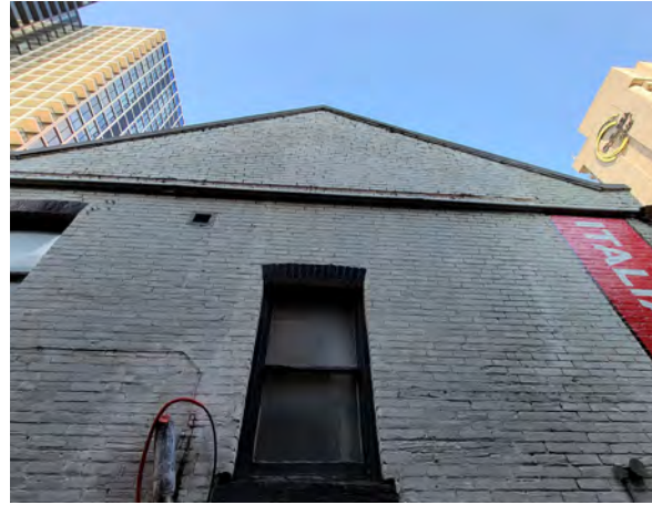
Figure 46: Third floor brickwork missing mortar and defective in condition (ERA, 2022).
