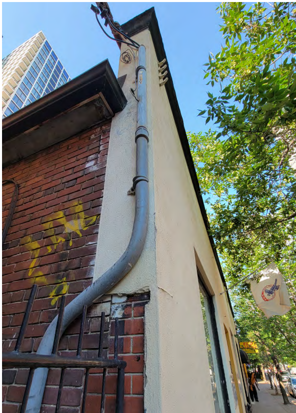
Figure 69: Parping with parapet wall is in poor condition (ERA, 2022).
