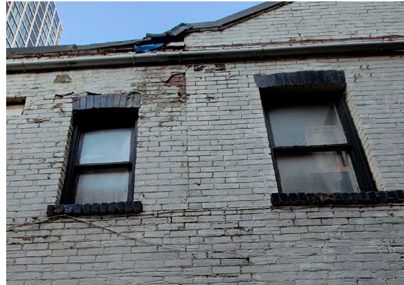
Figure 47: Wood windows, deteriorated brickwork in poor condition (ERA, 2022).
