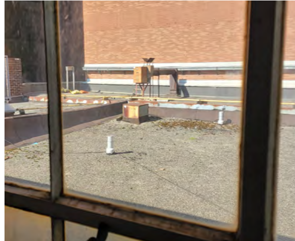
Figure 74: Painted metal flashing and pebble finish roof in poor condition (ERA, 2022).
